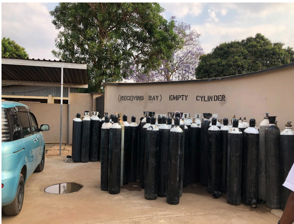
Oxygen cylinders at Kamuzu Central Hospital’s PSA plant, Lilongwe, Malawi, September 2023.
